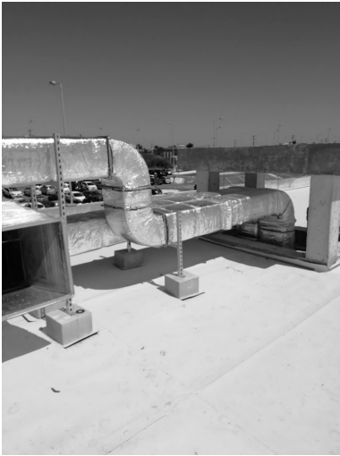
DELTA DUCT DERMITZAKIS Kos Airport
